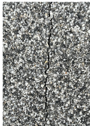
Example of cracking in resin bound.
